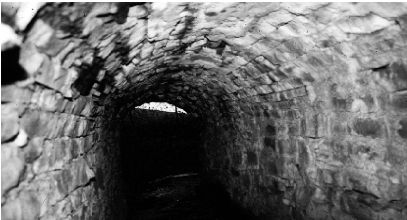
Figure 5. Superbly constructed culvert under the abandoned road from Doune to the Fords of Frew.
