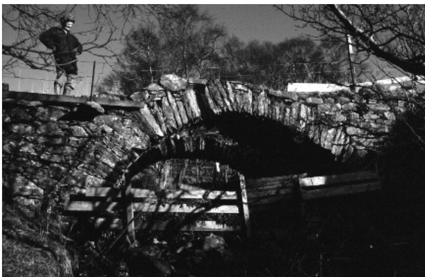
Figure 10. Bridge carrying the Military Road to Fort William, north of St. Bride's Chapel, Anie.
