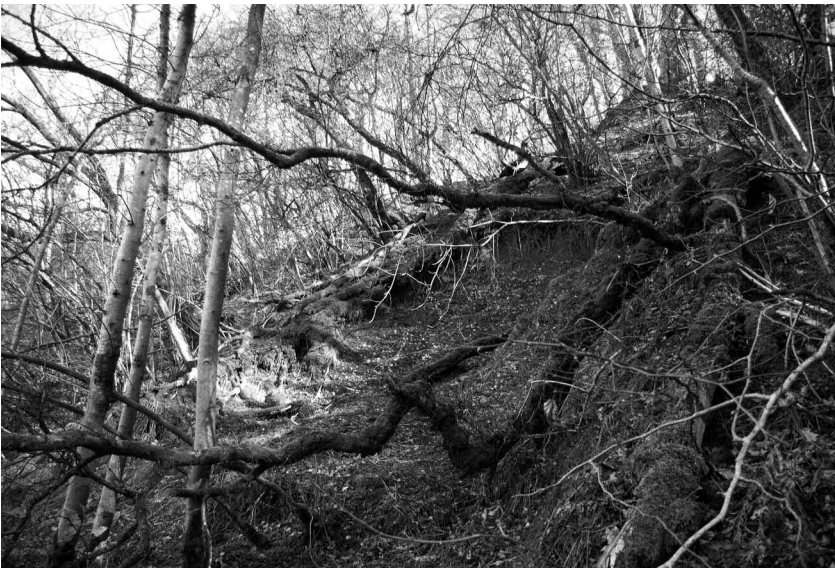
Figure 6. Slope failure above the roadway, near the crest of the slope, is unrelated to the existence of the road. Many such failures can be seen on both sides of the Glen, and they reflect the wider slope instability in Kippenrait Glen (photo march 2006).
