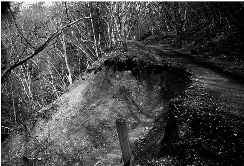
Figure 3. Head scar of the largest landslide photographed in April 1999: 2-3 m of substratum and nearly half the original road width was lost in this event.
