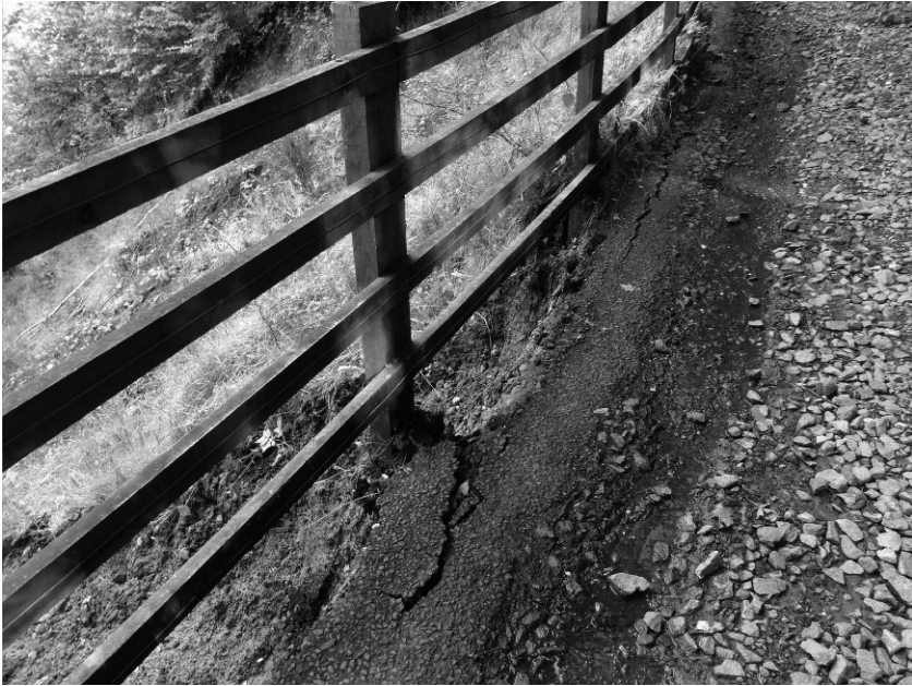
Figure 2b. Exposure of fence posts and cracking of tarmac at location of 2a.
