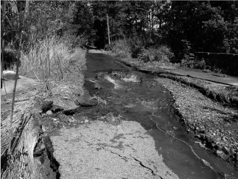
Figure 3a. Disruption of tarmac on the Glen Road.
